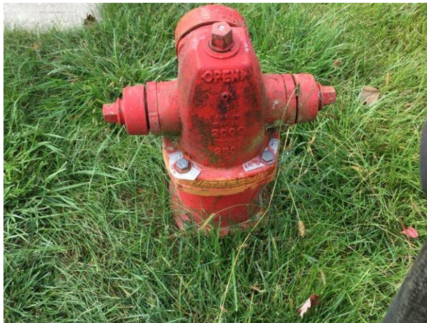
Hydrant. Taken so Year and Manufacturer is shown.
